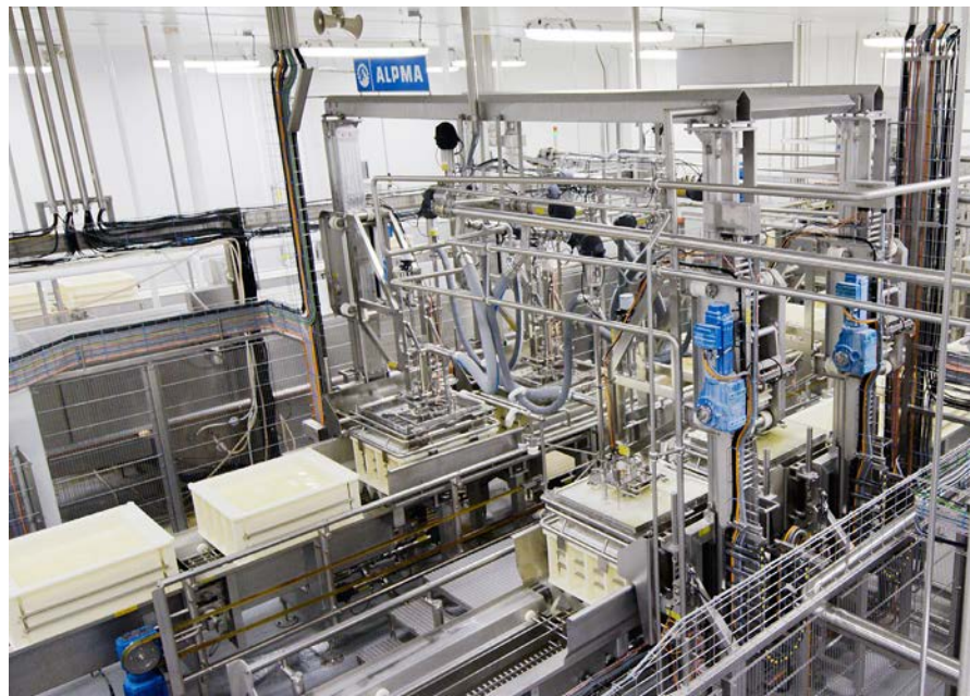
Luana’s latest expansions include a new process room. The Alpma system fills the 200-pound cheese moulds with curd, presses the block, cures, and then de-moulds the cheese before hitting the brine.
