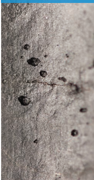
Corrosion, cracking, and pitting in 316 stainless steel pipe that has been etched with acid. Pits, cracks, and fissures may become attachment sites for biofilms.
